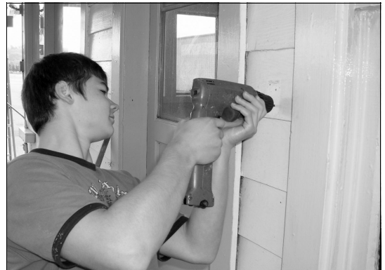
C/A1C Ivan Weber works on the building during the clean-up day at the Airport. Photo taken by C/CMSgt Jonathan Peterson
